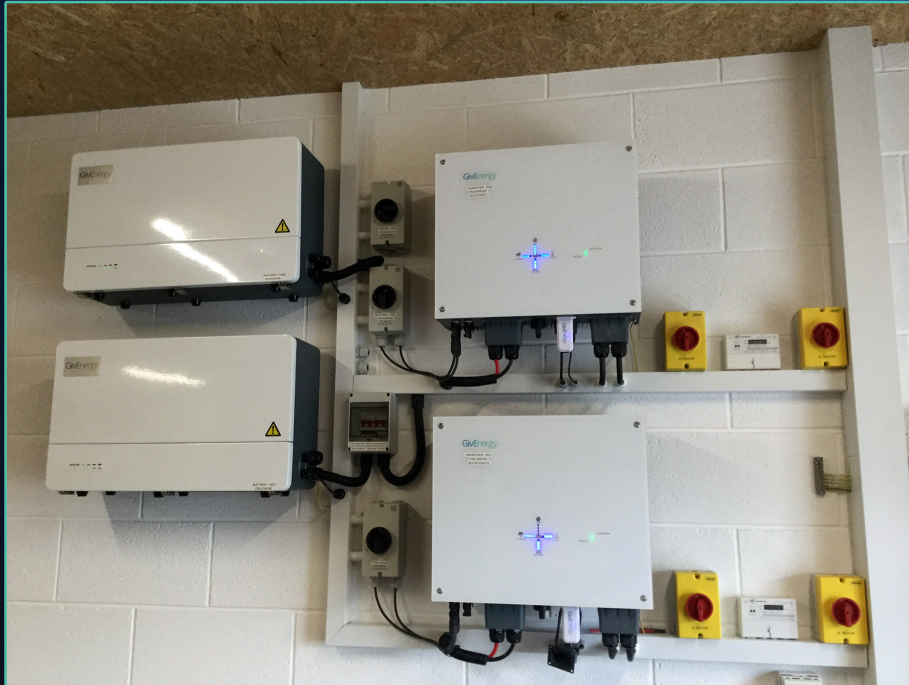
2 x 5kWh Hybrid Inverter 2 x 6.3kWh Battery
